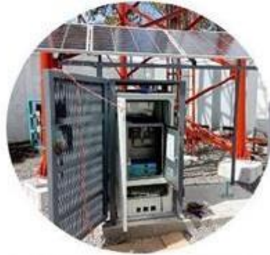
ISOLATED SOLAR GENERATION
